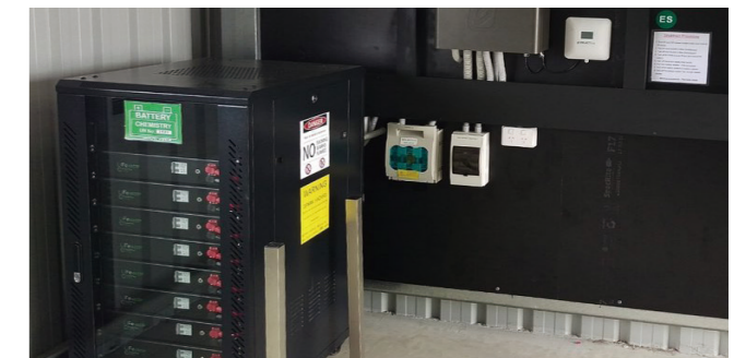
Rack-mounted lithium battery
